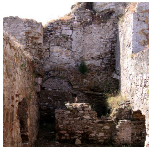
Fig. 4- Loredan bastion. Remnants of a previous wall with merlons and arched wall-walk.
