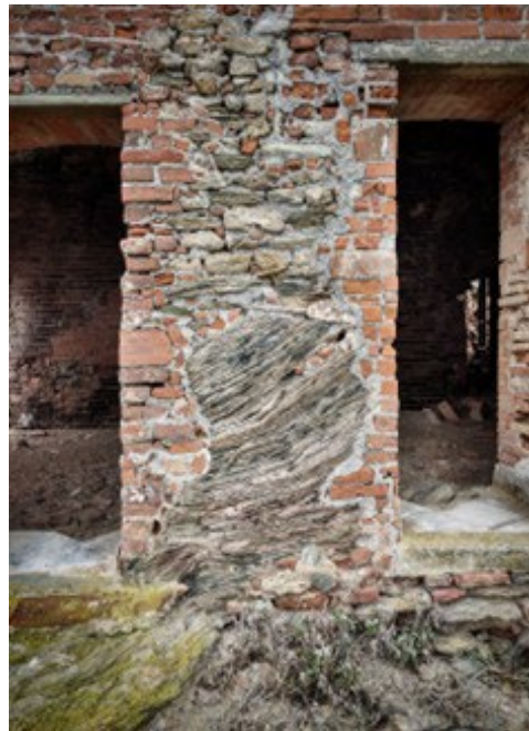
Fig. 4- Stone from the cliff merged into the masonry work at the upper base of the tower (photo by the authors, 2024).
