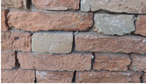
Fig. 15- Erosion of mortar joints, San Rocco fort (photo by Fabio Fratini, 2024).
