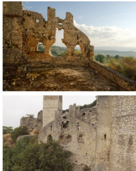
Fig. 7- Image of the two sides of the church still visible (graphic elaboration by authors, year).
