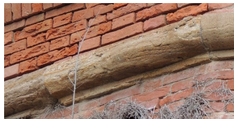
Fig. 10- Stringcourse in Pietra Panchina, Bibbona fort. Exfoliation phenomena in ashlar laid with the layering parallel to the surface of the masonry (photo by Fabio Fratini, 2024).
