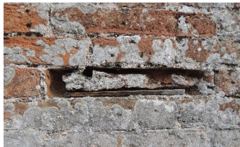
Fig. 14- Brick erosion and biological growth, San Rocco fort (photo by Fabio Fratini, 2024)
